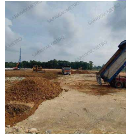
Earth filling works as part of Advanced Works Package at Rembus Depot
